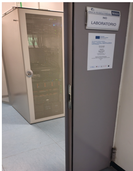
Entrance of the HPC INO lab at AdR CNR-FI
